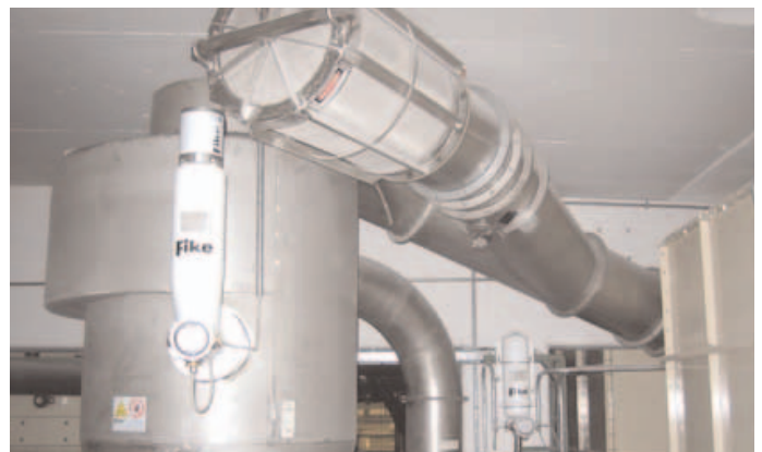
Inert Gas Suppression Container in indoor dust collector (Photo courtesy of Fike Corporation)
